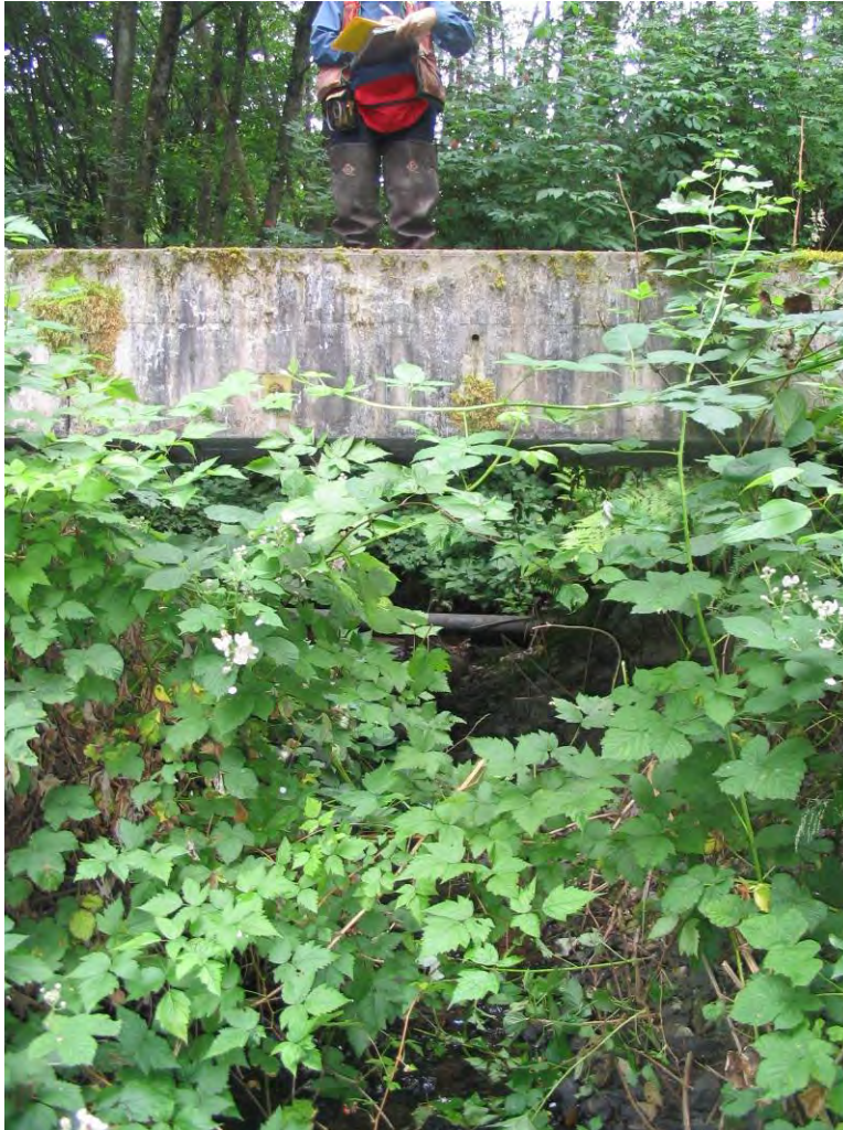
Figure 41. Sixteen Lake Camp Road, note exposed sewer main in middle of picture
