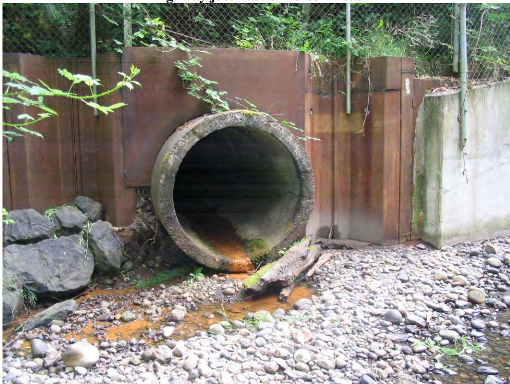
Figure 39. Looking upstream at old culvert (now overflow culvert) on Bulson Creek on Lake McMurray Highway just East of Bulson Road
