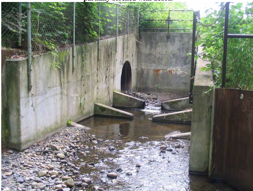
Figure 37. Looking at new replacement culvert on Bulson Creek on Lake McMurray Highway just East of Bulson Road
