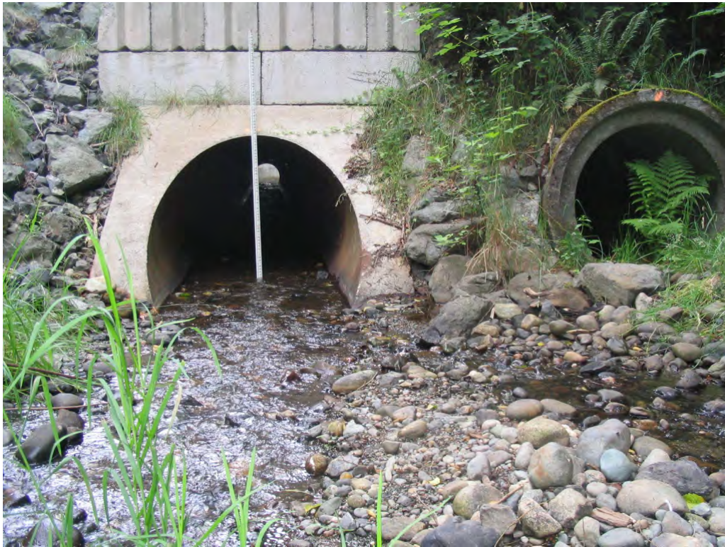
Figure 38. Looking downstream at new replacement culvert on Bulson Creek on Lake McMurray Highway just East of Bulson Road
