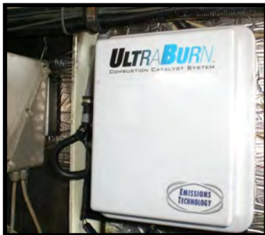
Main Engine #2 – Unit Mounting
