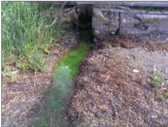
Figure 3. A positive septic system dye test at a house previously indicated by Crush.
