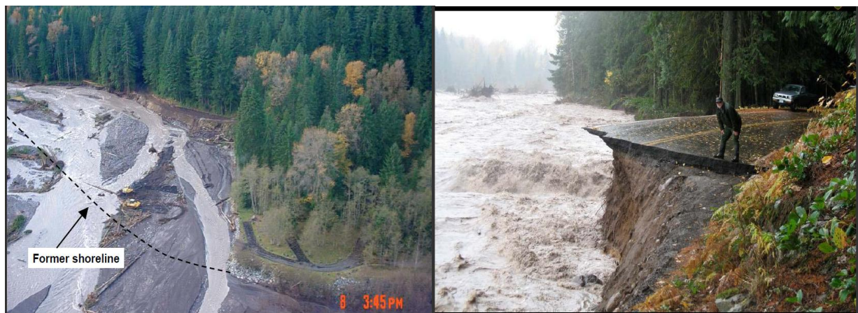
Figure 6.3 The flood damage at Mount Rainier National Park in November 2006: the Nisqually River at Sunshine Point (left panel) and the broken edge of the Nisqually road (right panel) (URL 5).
