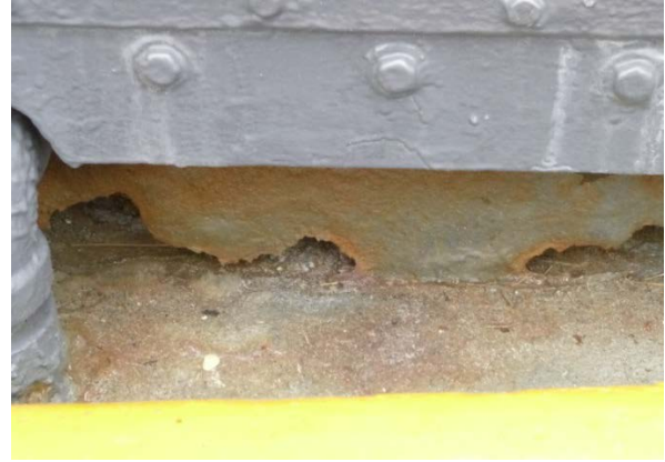
Figure 9: Structure at Engine Housing Base
