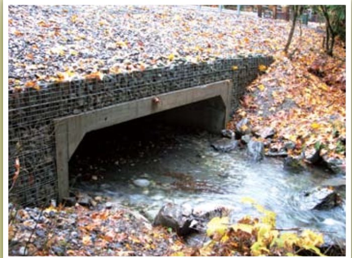
A new culvert at Gravel Creek: This culvert allows fish to swim upstream easily. It is also able to manage the flow of water that may come with rising water levels.
