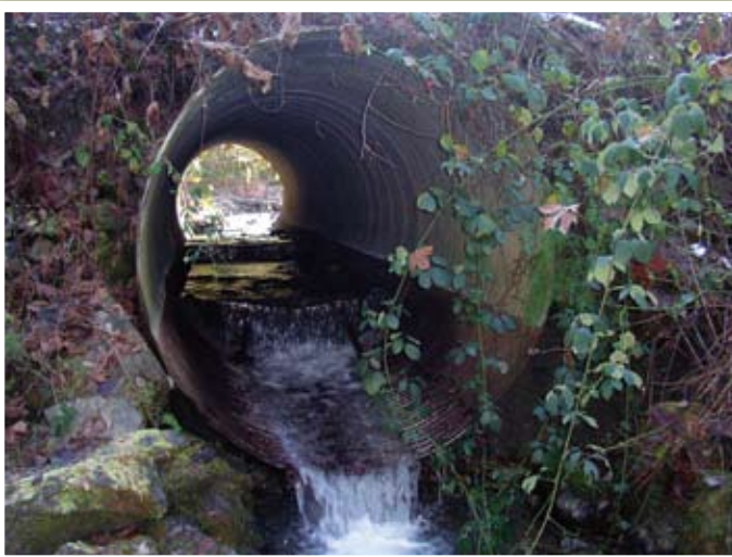
An old culvert at Gravel Creek: This culvert acts as a barrier for fish migrating upstream as the fish are forced to jump up and into the culvert to pass through.
